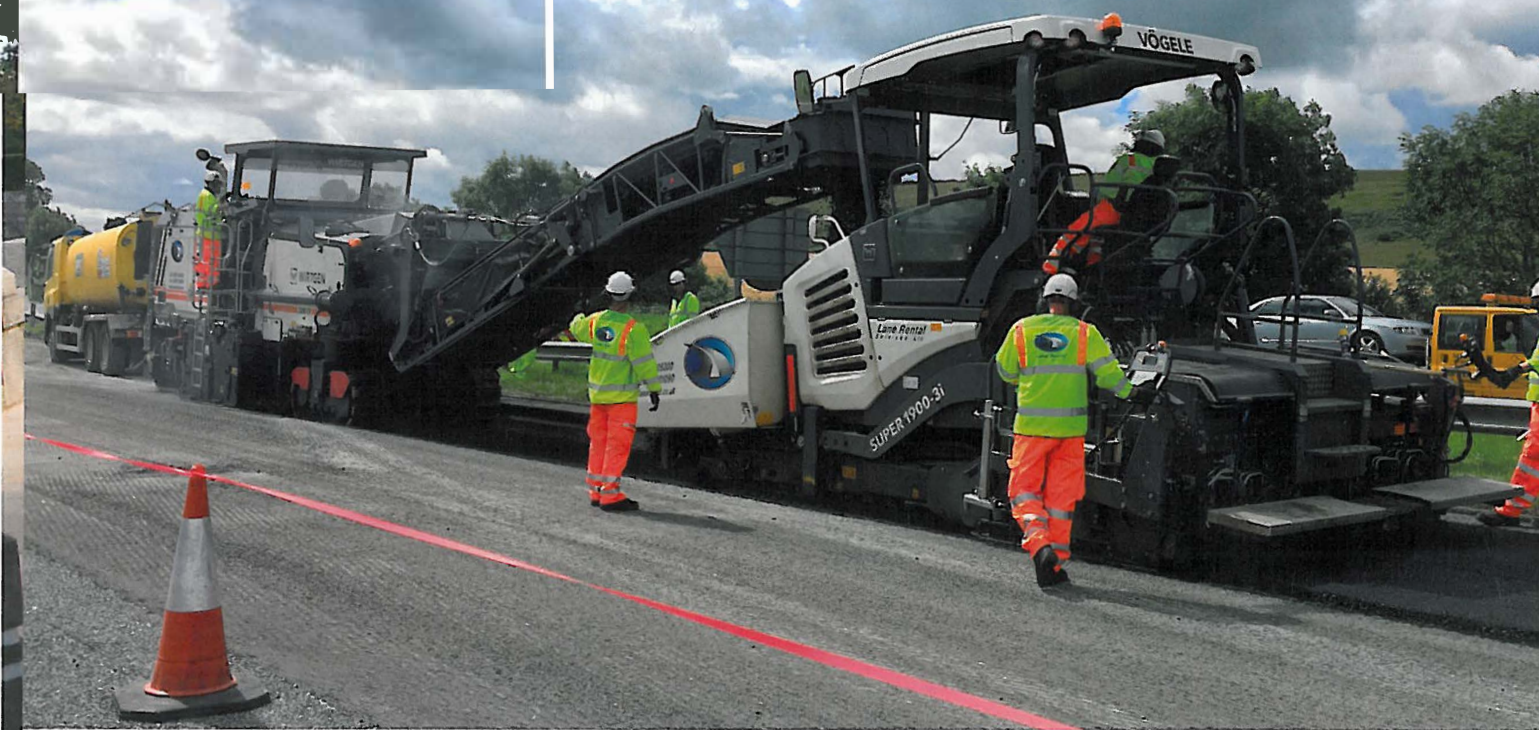
↑ Operatives work beside a paver receiving rejuvenated material from a conveyor attached to a Wirtgen machine directly in front
